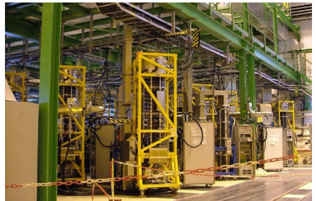
Fig. 10: LHC klystron gallery. TH2167 klystrons (in yellow support frames), WR2300 size waveguide system and racks with electronics are visible.
