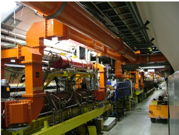
Fig. 8: The SPS RF cavities in the SPS tunnel. Front 800 MHz system (supplied by waveguides), further in the tunnel 200 MHz system (supplied by the coaxial lines)
